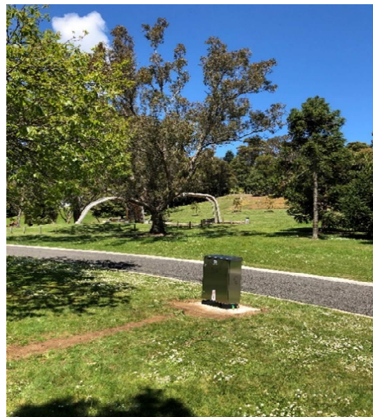
Figure 19: Power outlet at roadside
